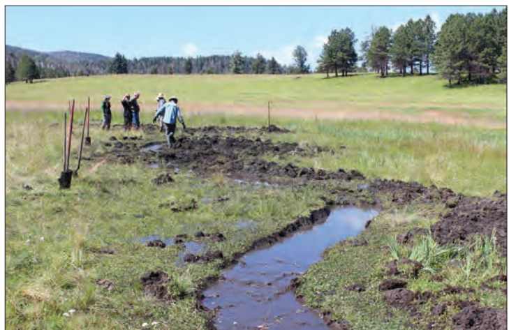
Figure 45. Site 20, July 2015. Worm ditch hand-dug by volunteers. Here water spills as sheetflow to the left. (©K. Menetrey, NMED)
