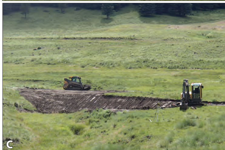
Figure 22. Site 52, August 3, 2016. A: Stockpiled sod. B: Excavator borrowing soil from pond. Skid loader is building and compacting the plug. Outlet in the foreground. C: Adding stockpiled sod to the surface of the plug. (©S. Vrooman)
