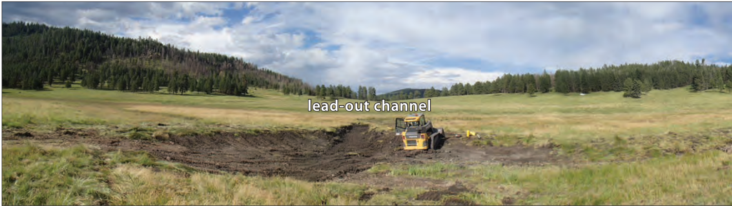
Figure 29. Sod has been added to cap the plug. Skid loader is constructing lead-out channel. (©S. Vrooman)
