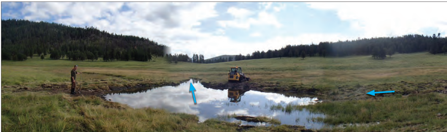
Figure 31. Construction completed and water from lead-out channel is spilling onto reconnected wetland surface. (©S. Vrooman)
