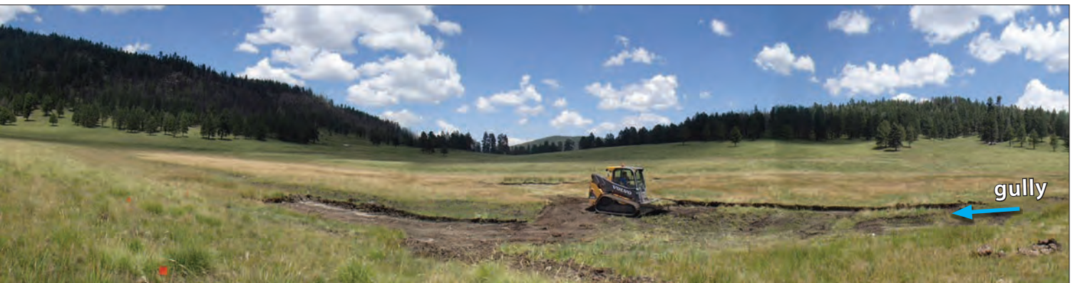
Figure 27. Excavator is removing sod from the surface of the area to be ponded and stockpiling it for surfacing the plug. (©S. Vrooman)
