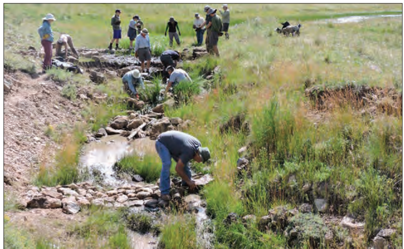
Figure 56. Site 50 and 51, July 18, 2015. Volunteers build grade control rock structures at stock pond outlet. (©W.D. Zeedyk)
