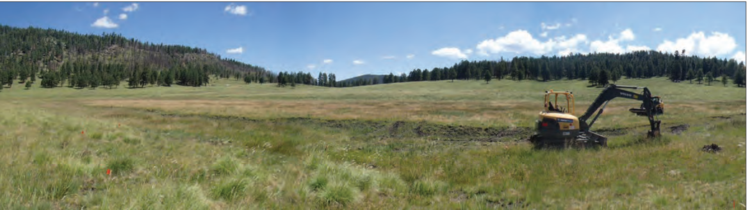
Figure 26. Beginning construction of the pond by borrowing fill for the plug. (©S. Vrooman)
